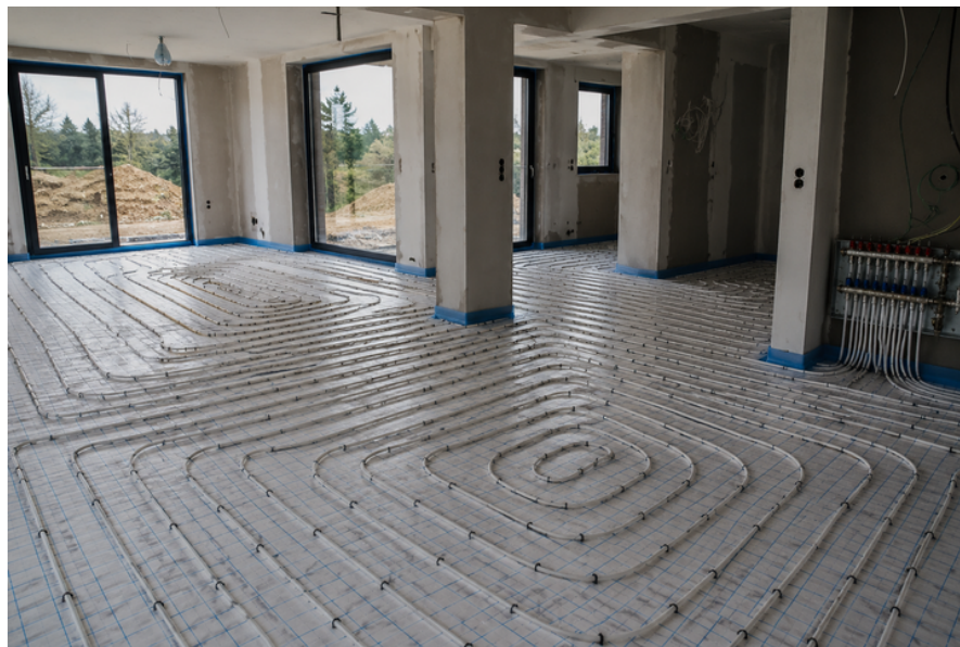
04 Radiant Underfloor Heating & Cooling
