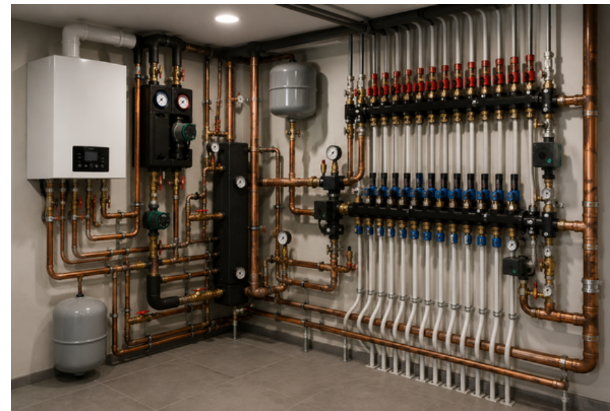
05 Hydronic Distribution Systems
